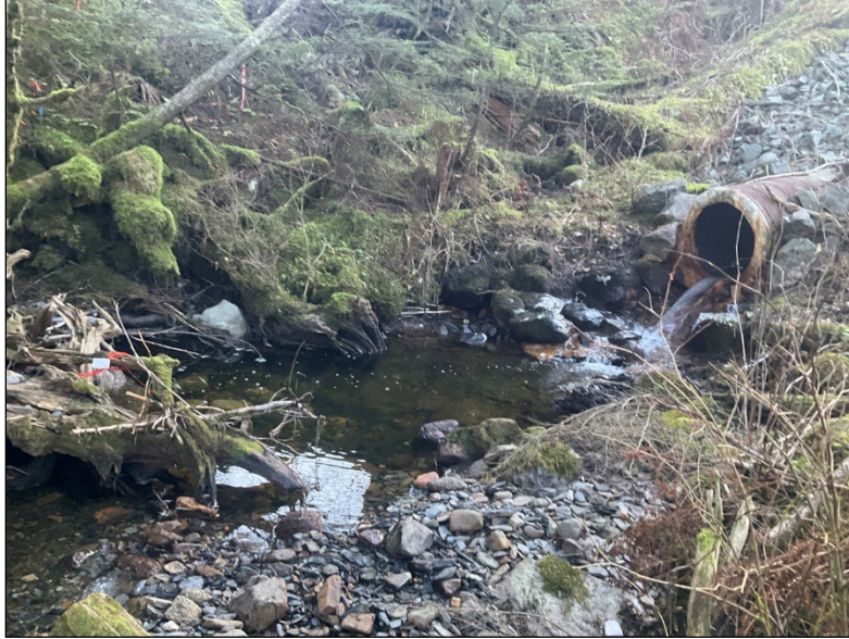
Figure 1.—Perched culvert outlet and pool at waypoint 1068.
