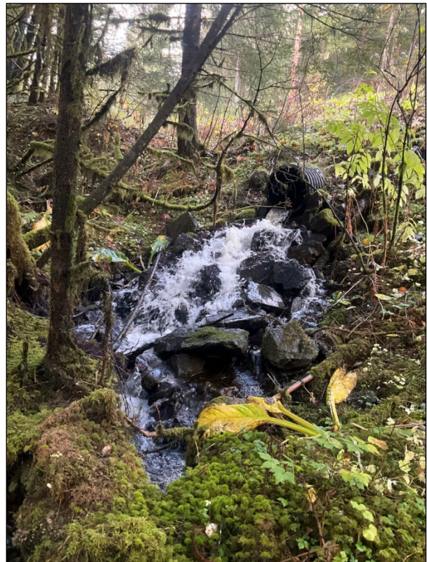
Figure 3.—Perched culvert outlet at waypoint 1034.
