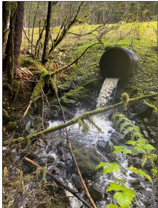
Figure 3.—Perched culvert outlet at waypoint 1030.
