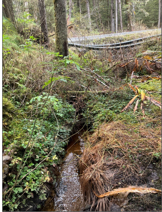
Figure 3.—Overcrowded channel just downstream of culvert outlet at waypoint 1041.
