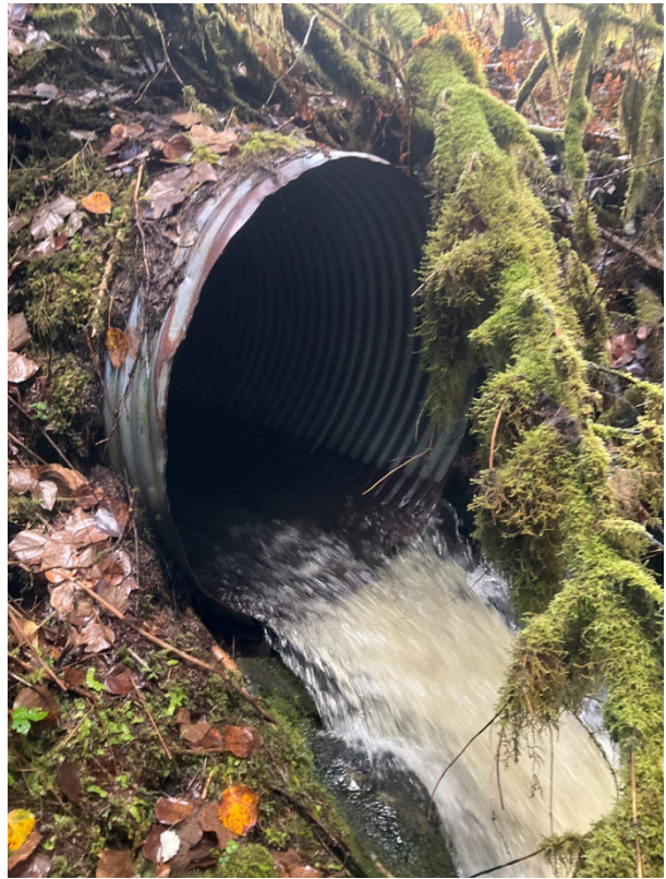
Figure 3.—Perched culvert outlet at waypoint 1036.
