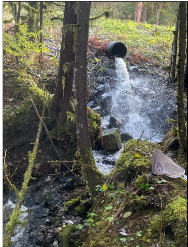
Figure 3.—Perched culvert outlet and conveyance stream at waypoint 1028.
